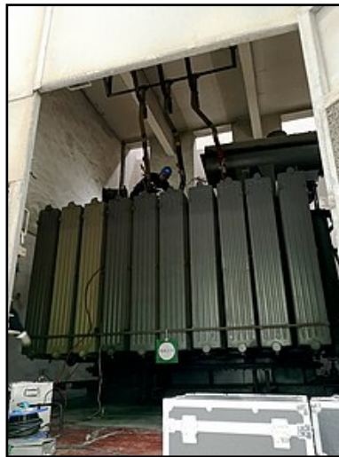
Substation transformer undergoing testing.
