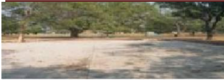
Figure-2: A view of PFRC used in parking over lean base concrete
