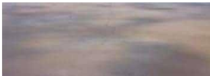
Figure-5: A closer view of crack due to no expansion joint
