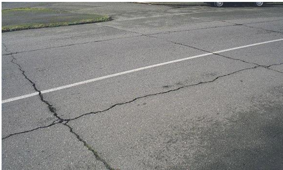
Figure 3.6 Joint Reflection Cracking
