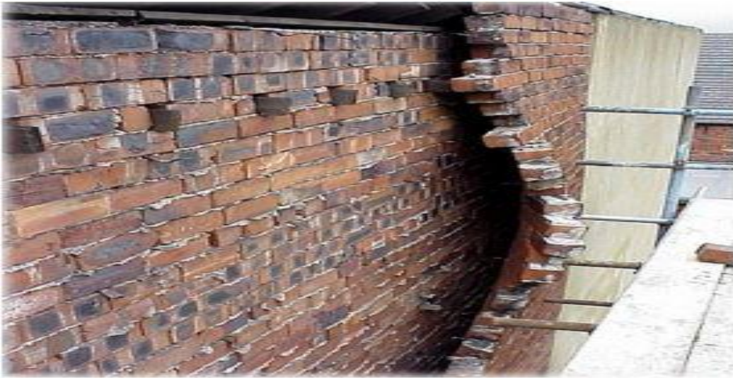
No Wall ties causing bowing and 'peeling'
