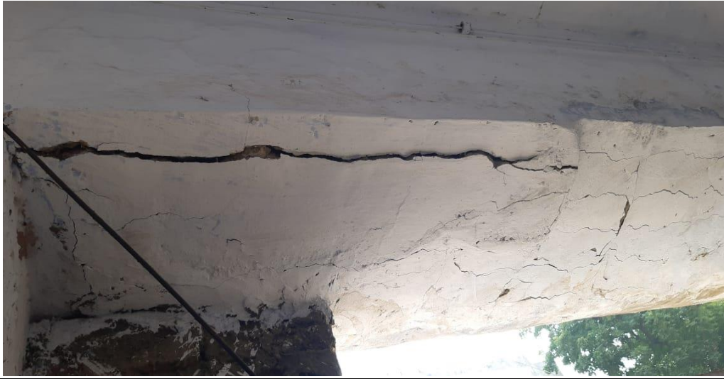
Fig: Picture of random cracks due to drying shrinkage
