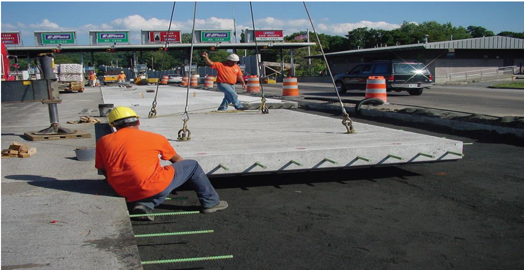
Figure 3.5. Placement of grade-supported precast panel for over-night use prior to installation of bedding grout
