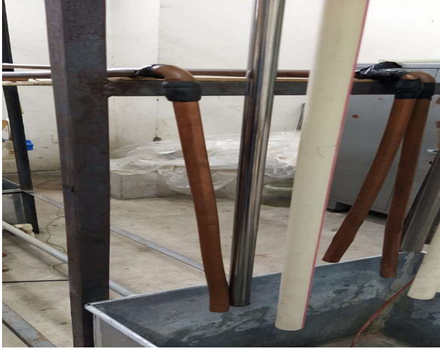
Fig: 3.3 Pipes and these materials used in the setup
