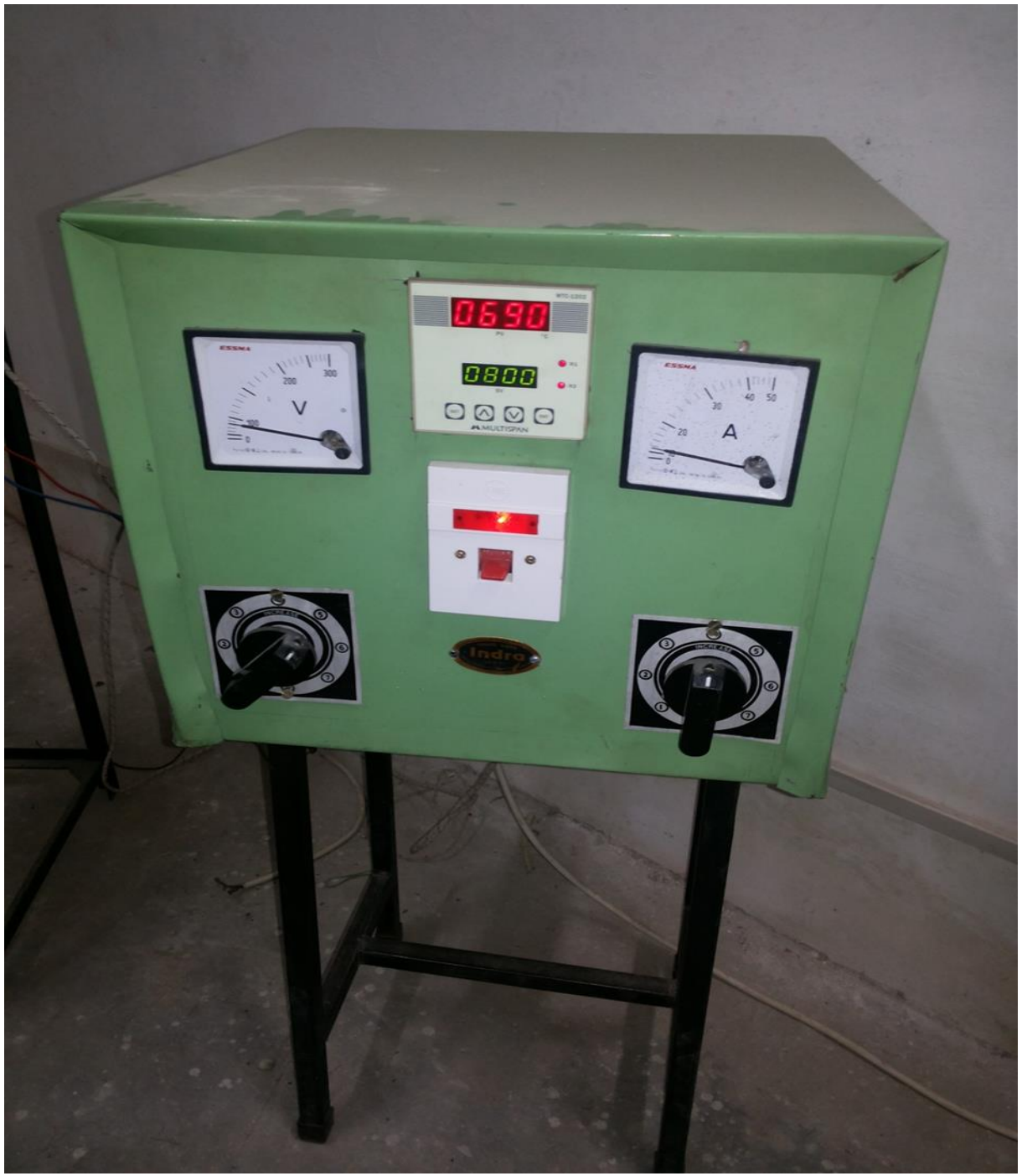
Figure. Heavy duty transformers
