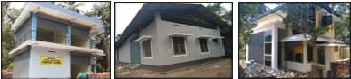
Figure 12 Construction of Marketing Center, Plastic Waste Management Unit & Counselling Centre for Teenage Girls
