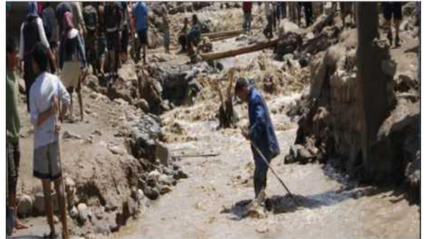
PHOTOGRAPH 4: SHOWING DAMAGE BY CLOUD BURST, 2010
