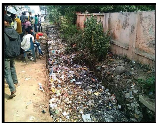
FIG 4.17 DRAINAGE CLOGGED , DELHI
