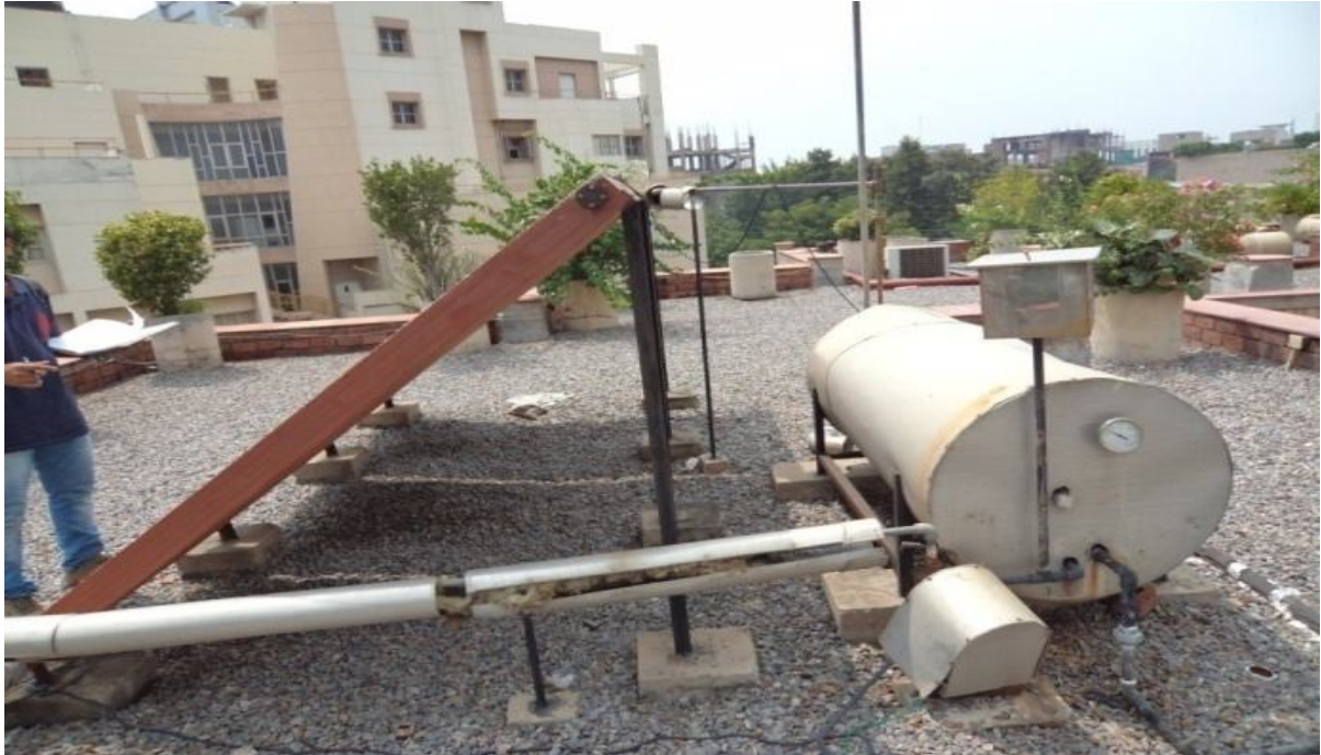
Figure 17. Solar Water Heater on the terrace
