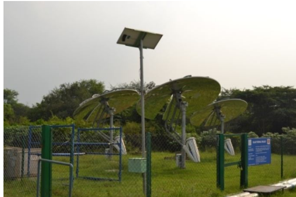
Figure 24. Solar thermal plant for power generation
