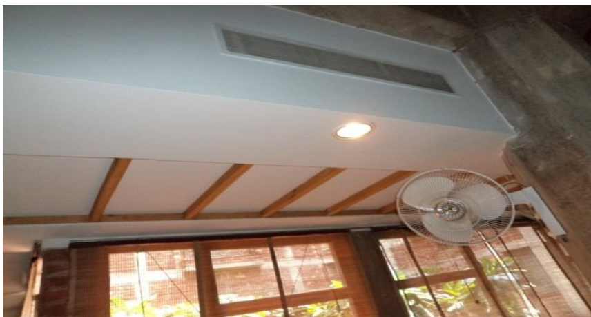
Figure 16. Evaporative Cooling Duct in the Library (Basement)
