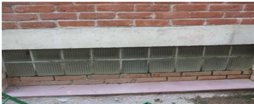
Figure 10. Glass bricks on East and West façade for Natural light in thebasement
